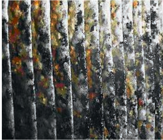
FIG. 22. Microbiological growth on tube surfaces.
